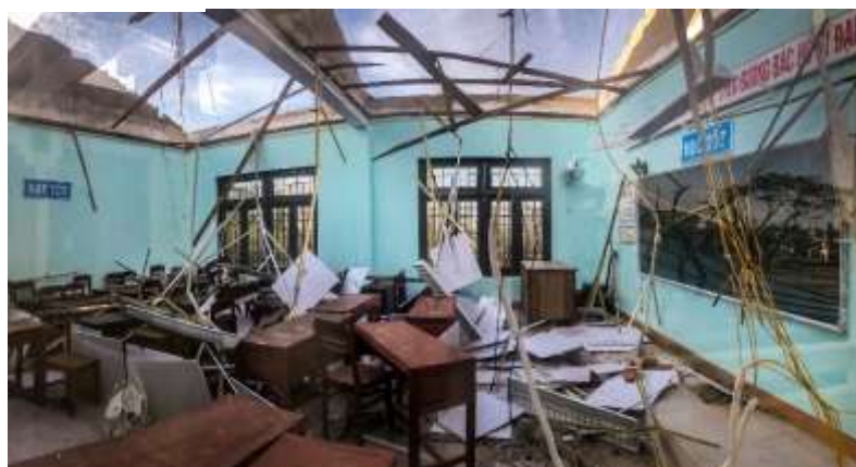
Broken school facilities inside a classroom without the roof at Vo Bam junior high school in Tinh Khe Commune, Son Tinh District, Quang Ngai Province on October 29, 2020.
