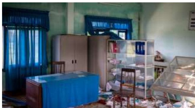
Broken health facilities at Tinh Khe primary school in Tinh Khe Commune, Son Tinh District, Quang Ngai Province on October 29, 2020.
